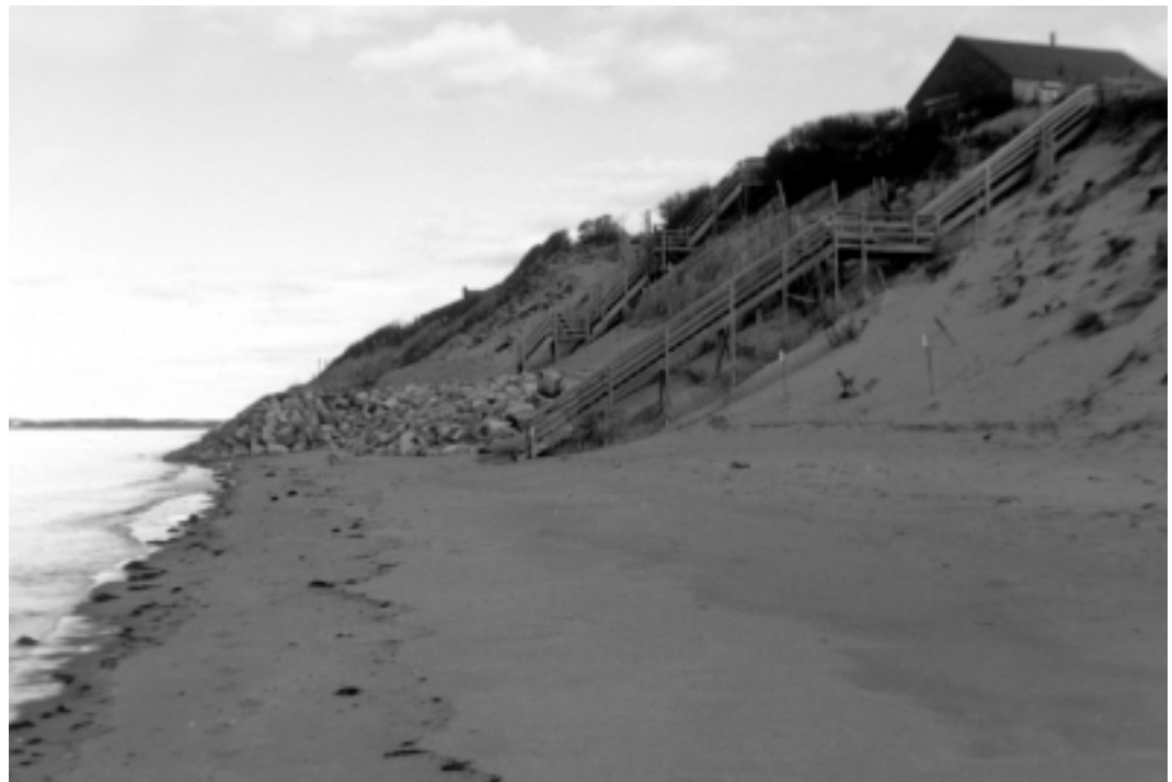
Revetment construction on an eroding coastal bank in Eastham, MA, has resulted in the loss of the coastal beach fronting the structure.
