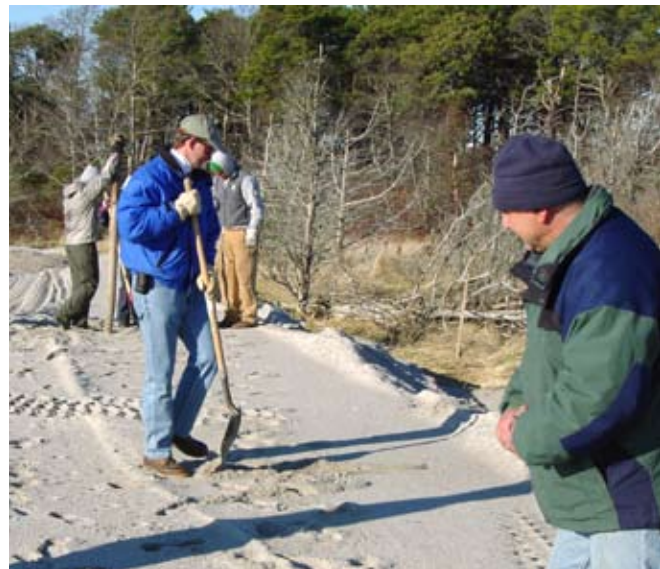
Figure 7. Ted Keon, Director of Coastal Resources for Chatham, Mass., uses a shovel for larger size holes for 6x8 poles while project manager Tim Friary looks on.
