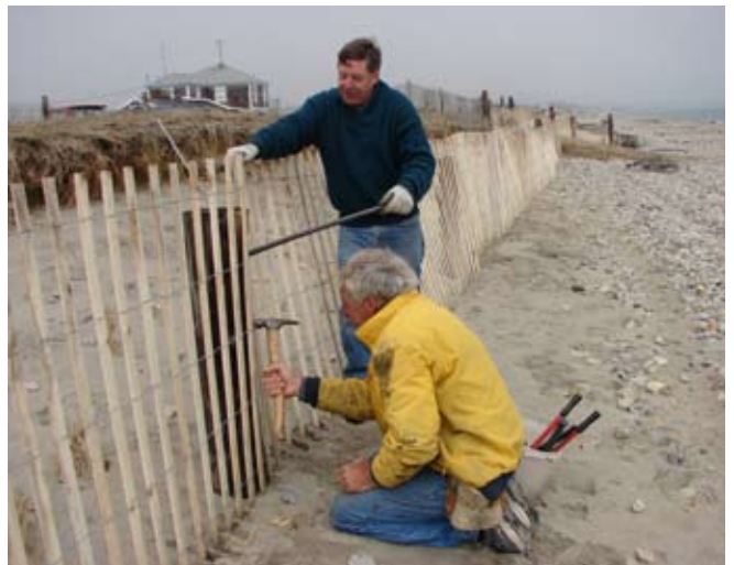
Figure 13. Experienced sand fence installers Joe Grady and Dick Sjosted attach fencing to posts. The snow fence is being held taut by a crow bar while a 2" galvanized staple is hammered into the post loosely attaching the snow fence 'wire' to the post.
