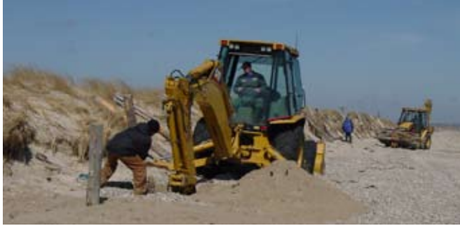
Figure 8. Using an excavator to dig larger size holes for 6" to 8" poles, Duxbury Beach, Mass.
