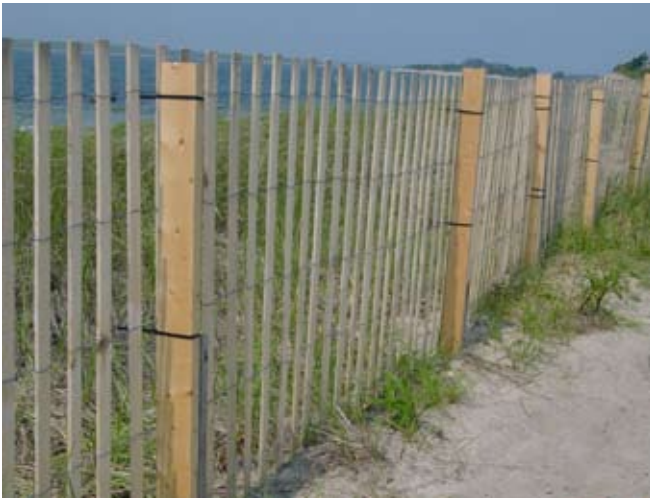
Figure 15. Sand/snow fence held to 2x4 posts with tie-wraps, an alternate method of installation.
