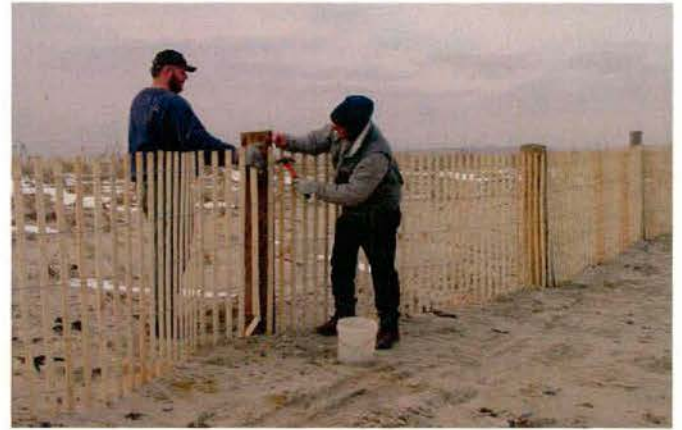
Figure 12. Fence is attached to 6" diameter posts.
