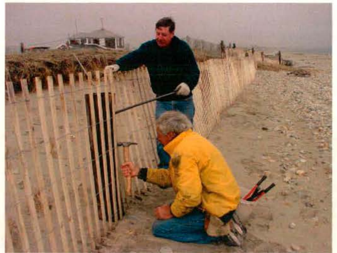
Figure 13. Experienced sand fence installers Joe Grady and Dick Sjosted attach fencing to posts. The snow fence is being held taut by a crow bar while a 2" galvanized staple is hammered into the post loosely attaching the snow fence 'wire' to the post.
