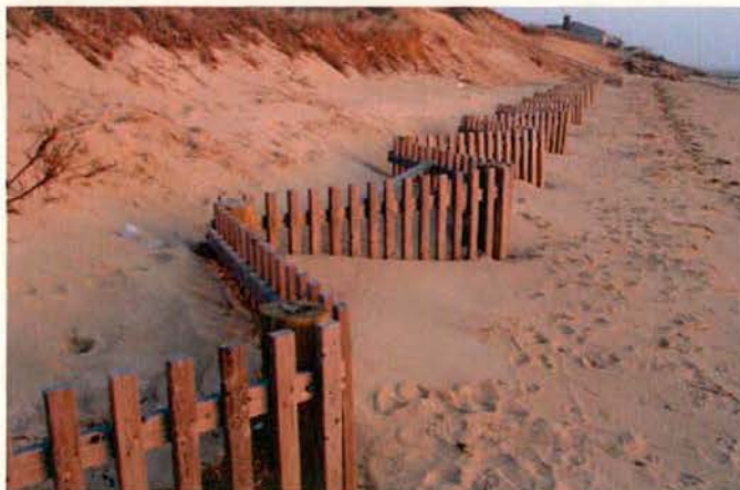
Figure 17. Sturdy sand drift fence made of 2x3 vertical and horizontal members, with 6" diameter posts.
