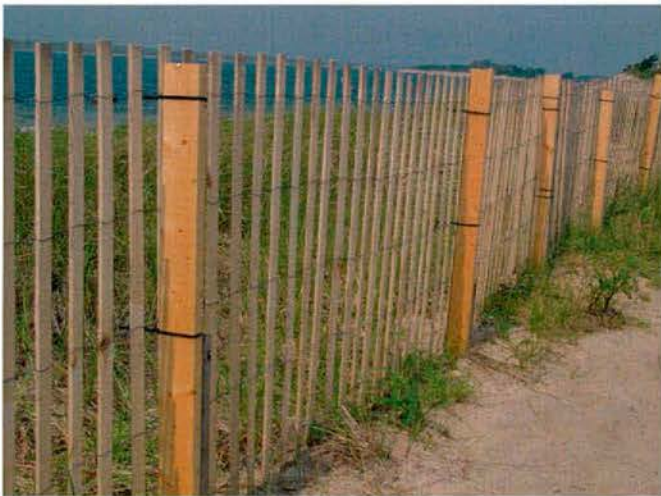
Figure 15. Sand/snow fence held to 2x4 posts with tie-wraps, an alternate method of installation.
