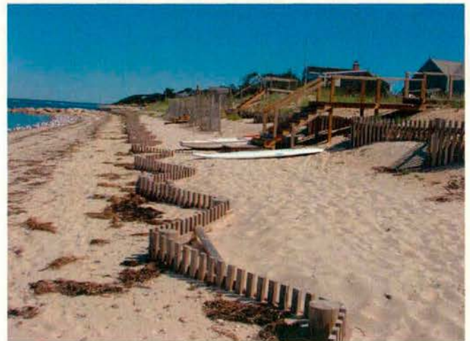
Figure 18. Double row of sturdy sand drift fence — made of 2x3 vertical and horizontal rows with 6" diameter posts which are partially buried when installed. This style of fence is generally used in areas of small waves or ice.
