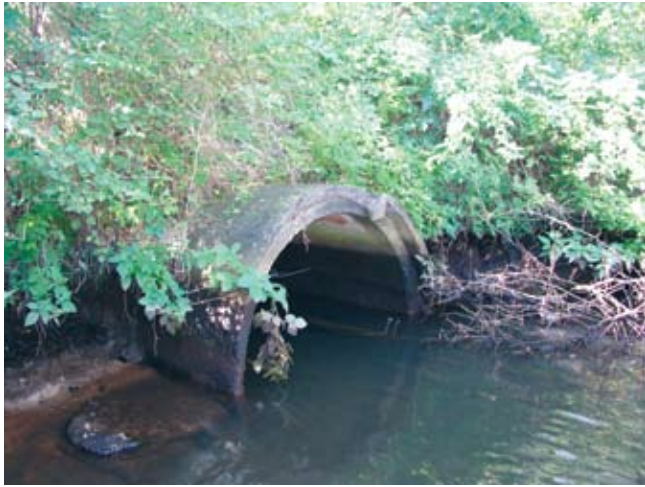
Restrictions like this culvert dramatically reduce tidal flow upstream.
