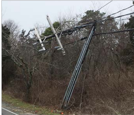
Figure 4-22. Downed or damaged power lines in a residential area can pose a serious danger to public safety. Image courtesy of CCCE/WHSG
