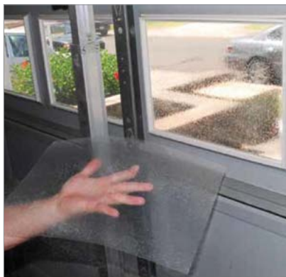
Fig 4-18. Laminated film comes in various thicknesses and strengths. Here the film is applied to an existing window before it is fastened to the frame with silicone structural sealant.
