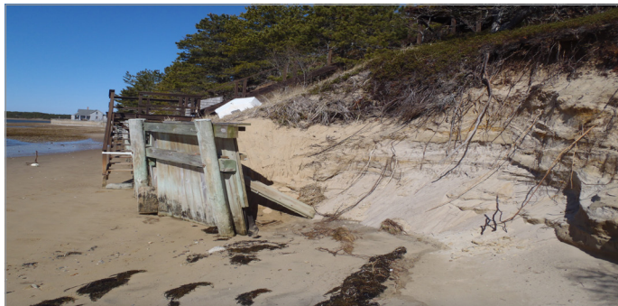
An example of scour at the end of a bulkhead. Waves refract around the terminus of the CES exacerbating the erosion and compromising the structure.
