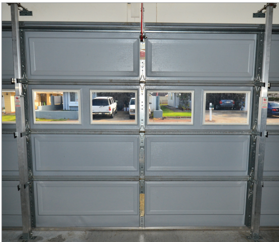
Figure 3-16. Vertical braces such as these can be deployed during high-wind events to strengthen the garage door. The braces are secured from the header over the garage door to the fasteners installed in the concrete floor. Deployment and breakdown are about 10 minutes each. The windows have been covered with a laminate film. Image courtesy of Dennis Hwang.
