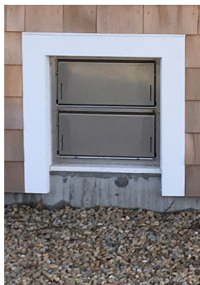
Figure 3-17. Image of flood vents courtesy of Cape Cod Commission
